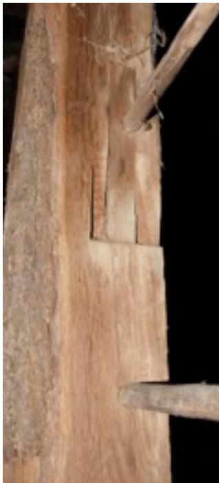
Filled mortise supporting the rung of a ladder. A red snap line aligns with this mortise.
